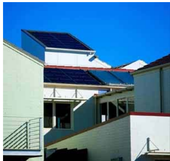
Panels on the roofs of the Athletes Village generated electricity and hot water.#
